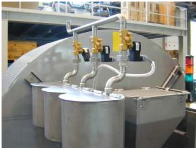
Chemical tanks with automatic dosing
