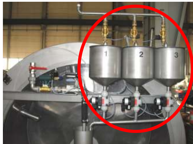
Chemical tank with automatic dosing
